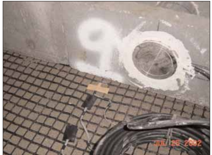
Earth Pressure Transducer Behind the Block and Strain Gages on the Geogrid
