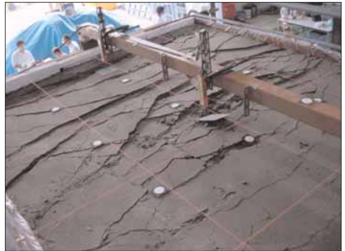
Surface Cracks at the Retained Soil
